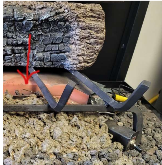
Figure 2 – Arrow pointing at pilot assembly
