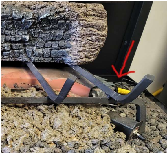
Figure 1 – Arrow pointing at pilot control knob with logs removed
